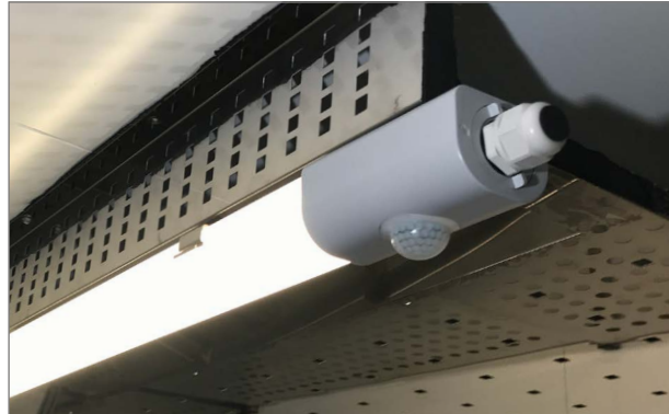
Lighting with motion sensor.
